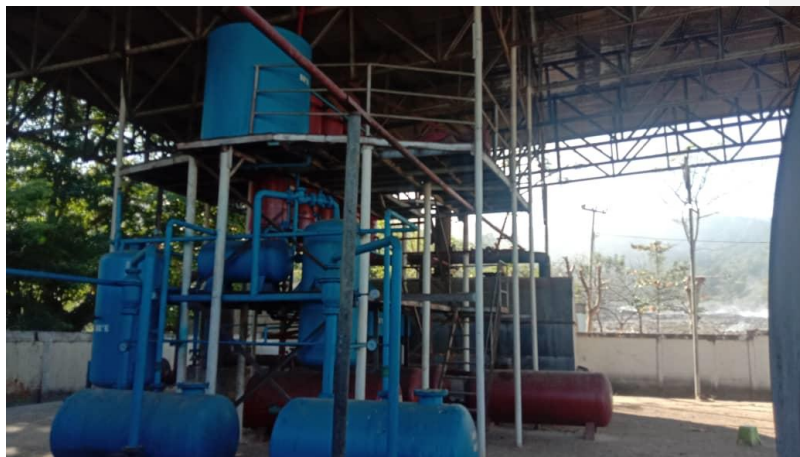
Figure 2 The current waste oil plant at Tibar, Timor-Leste. Pictures taken May 2021. ©COWI
