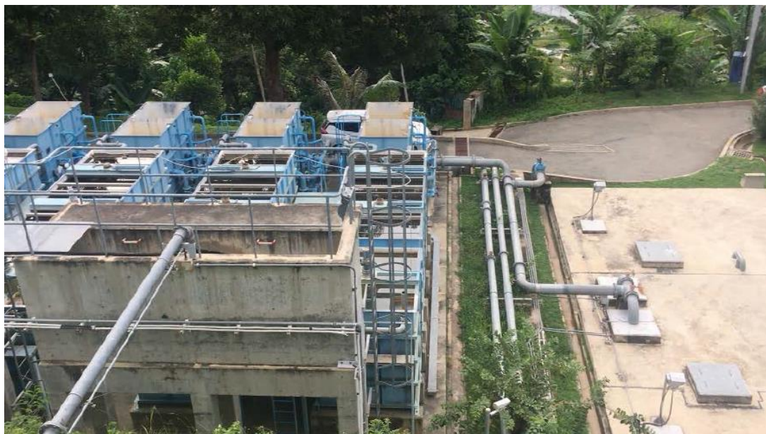
Figure 6. The four parallel treatment trains of the Bemos WTP
